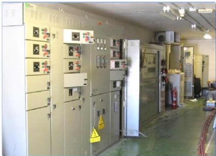
New electrical building
